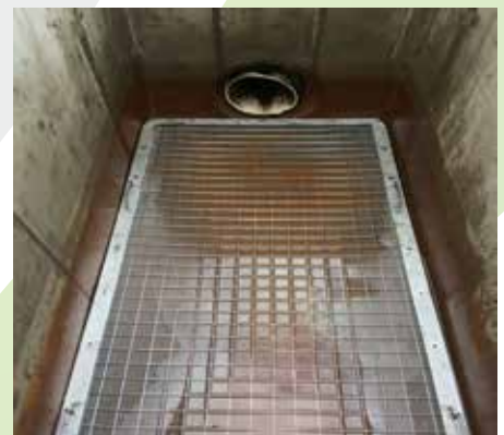
Secondary Treatment Chamber
