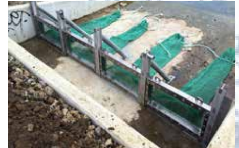
Figure 1 – Ecosol™ four module and constructed trash rack system.
